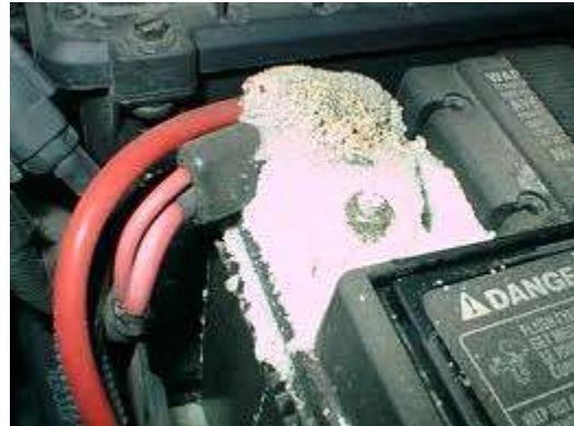
Sulphate deposit in terminals
